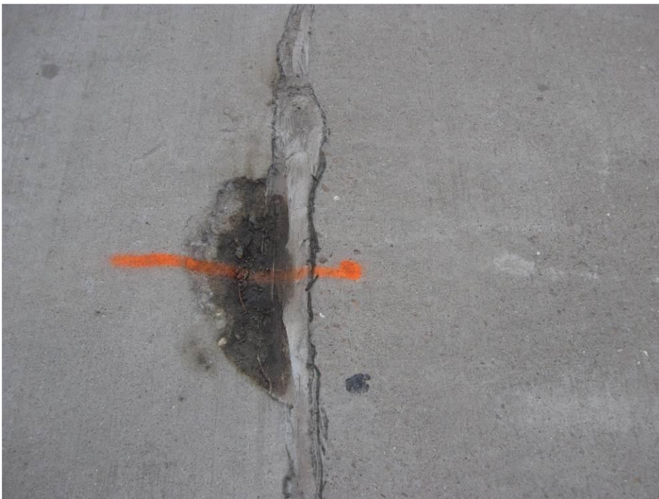
Photo 4 – typical floor spall over shear connector.
