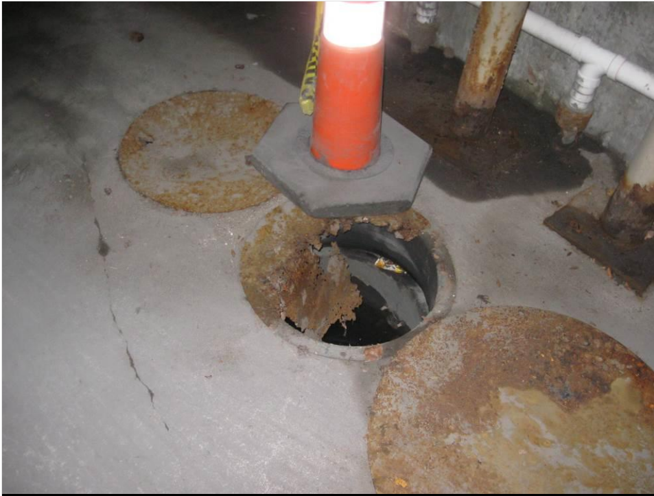
Photo 5 – Corroded cover on triple basin.
