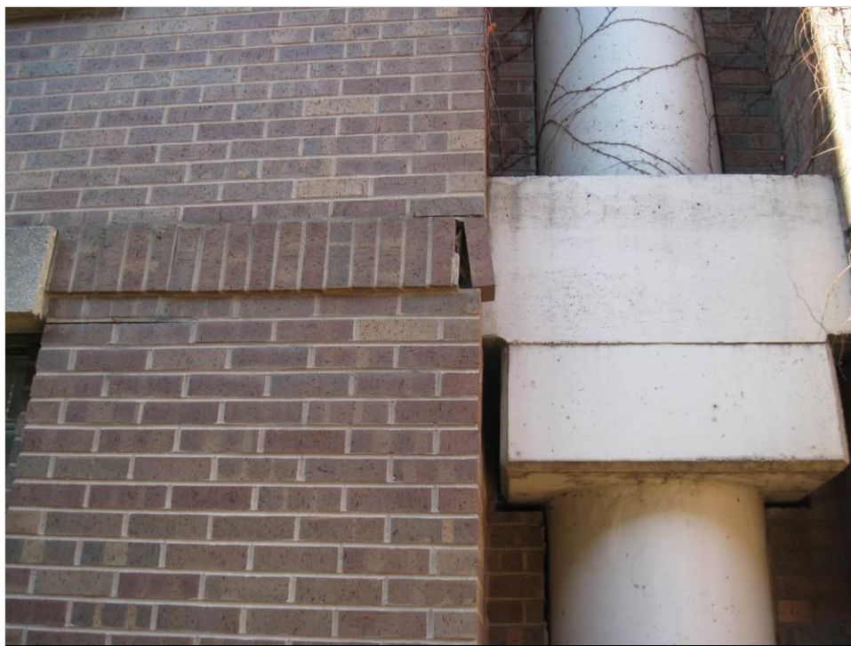
Photo 18 – Loose masonry on façade.
