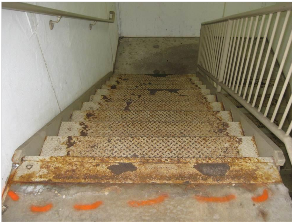
Photo 2 – Corroding stairs within stair tower.
