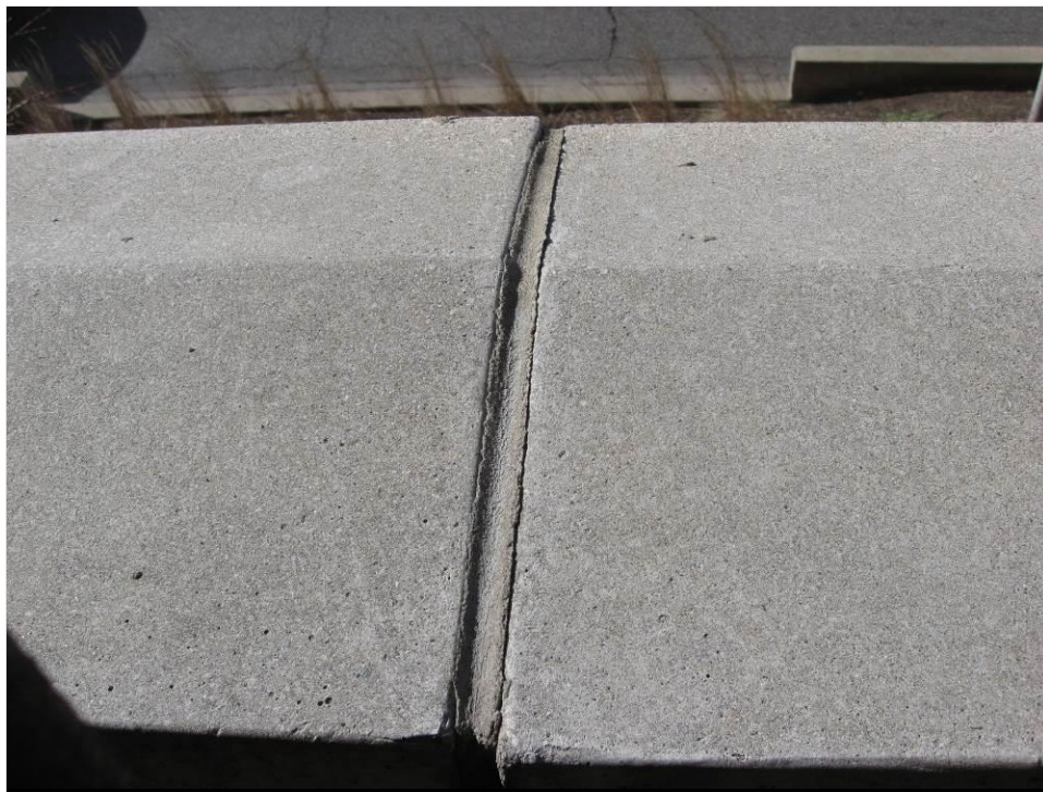
Photo 17 – Severely deteriorated mortar joint on cap stone.
