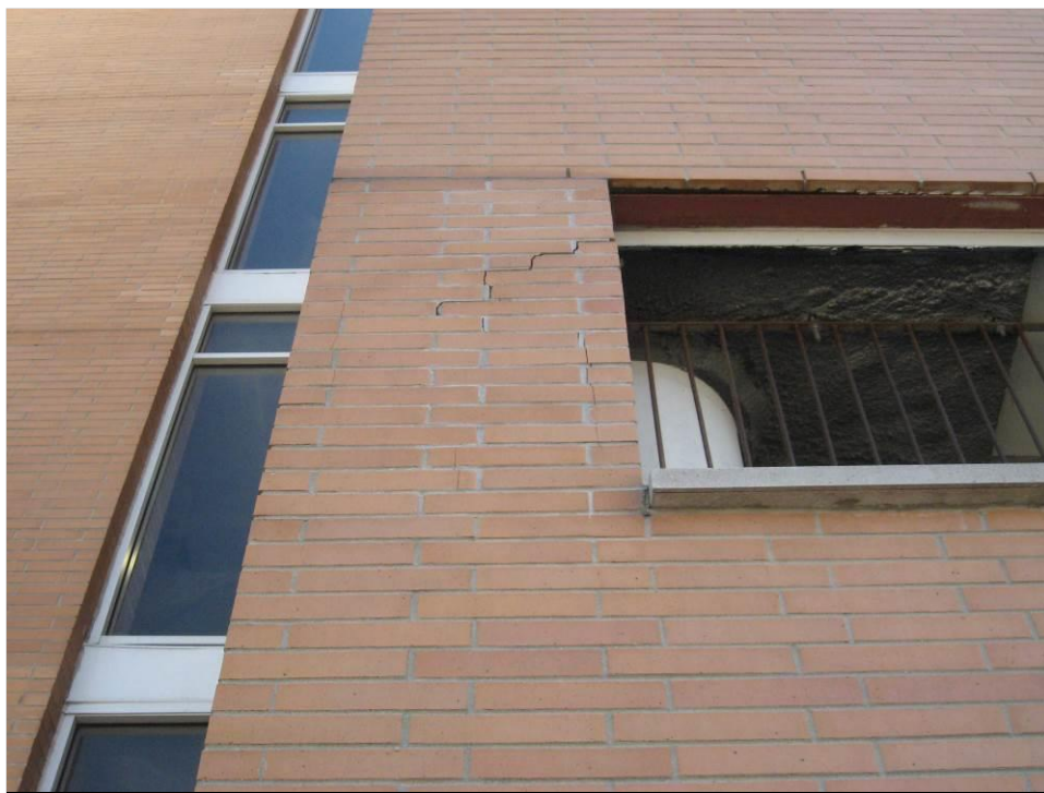
Photo 5 – Crack in masonry on façade.
