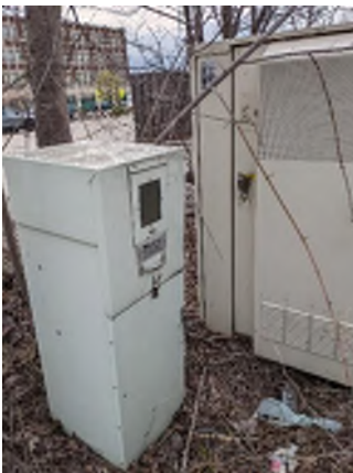
Southeast corner of property, transformers
