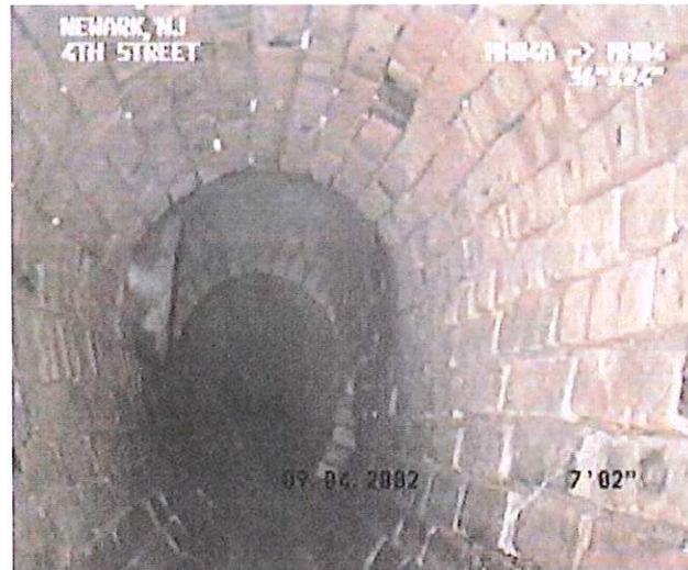
Figure 2. Example of Condition Grade 2 Brick Sewer- Minimal Potential for Short-Term Collapse; Further Deterioration Probable
