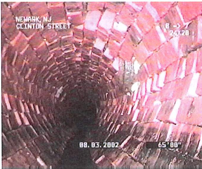
Figure 3. Example of Condition Grade 3 Brick Collapse Unlikely in Immediate Future; Further Deterioration Likely
