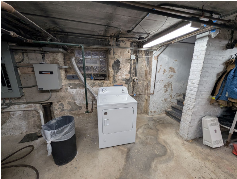
LOW CLEARANCES / POOR EQUIPMENT ACCESS
