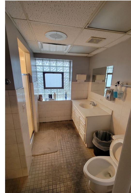
INSUFFICIENT TOILET FACILITIES
