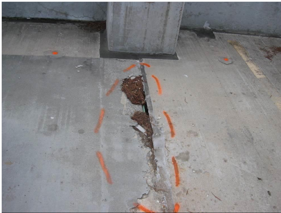
Photo 5 – Hole in the flange.
