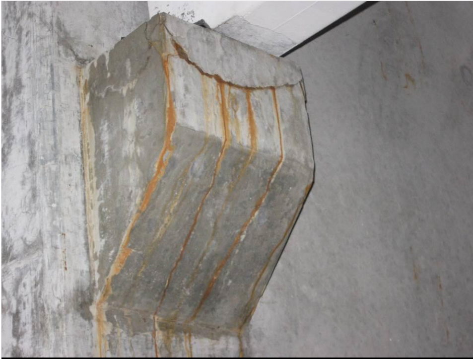
Photo 9 – typical concrete delamination at haunch for tee stem bearing.
