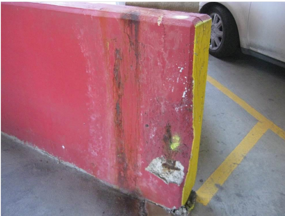
Photo 6 – Typical wall deterioration.
