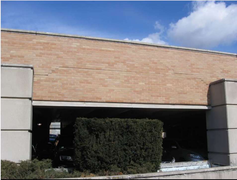
Photo 9 – Severely deteriorated masonry section on façade panel along south wall.
