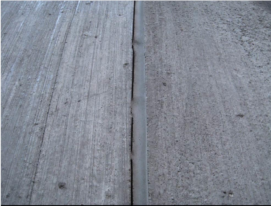
Photo 1 – Adhesion failure of tee-to-tee joint sealant.
