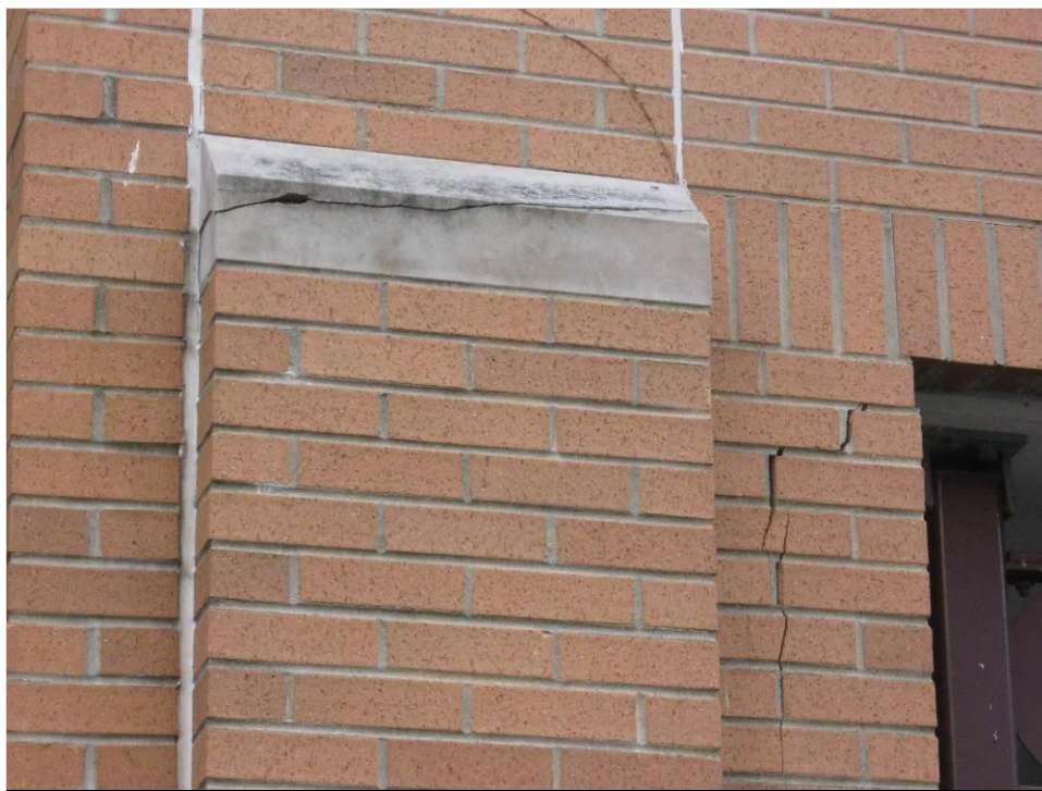
Photo 12 – Broken cap stone and cracked masonry.
