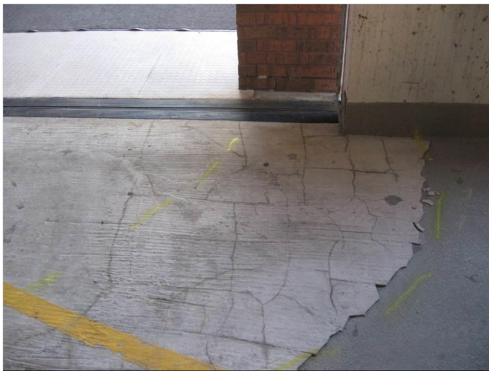
Photo 3 – Floor slab deterioration at entrance to elevator tower.
