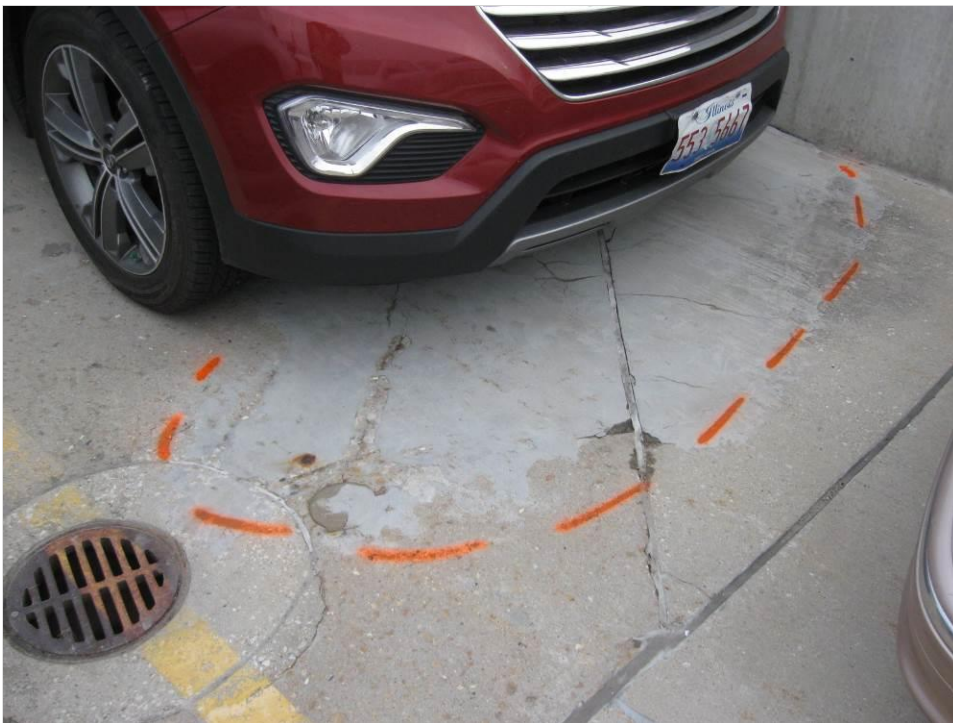
Photo 2 – Typical concrete delamination and deterioration at cast-in-place washes.
