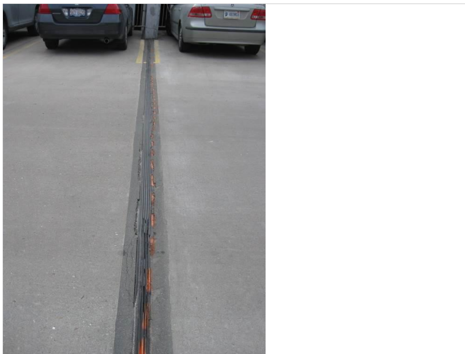
Photo 14 – Severely deteriorated expansion joint at grade slab.
