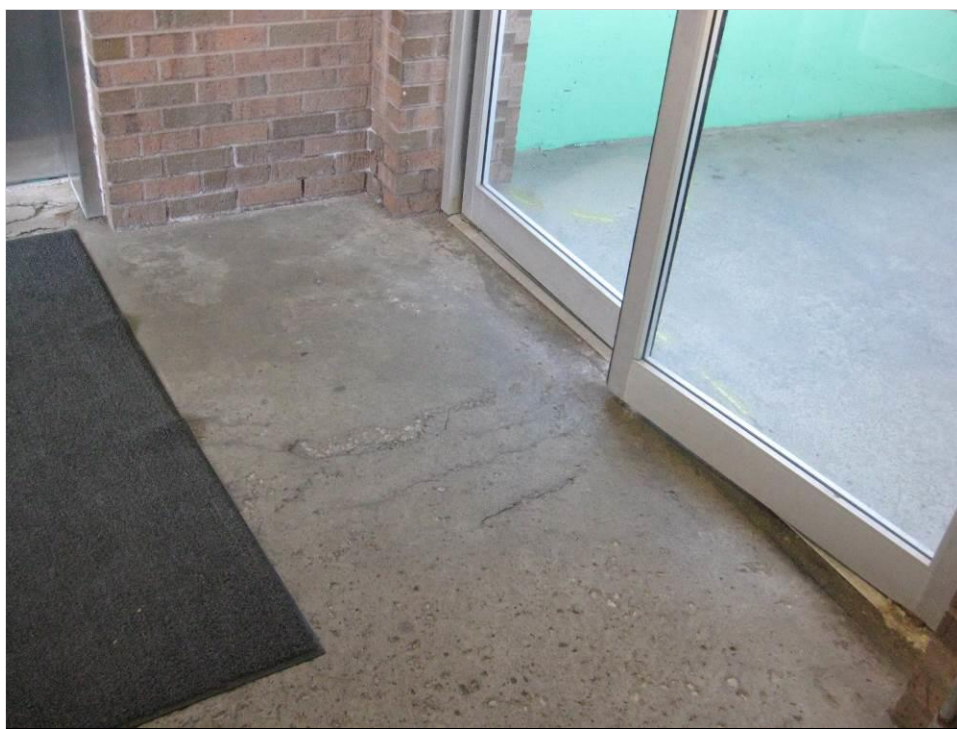
Photo 4 – Floor slab deterioration within stair/elevator tower.
