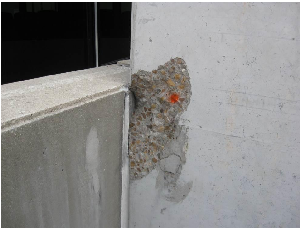
Photo 8 – Spall on the side of a column.
