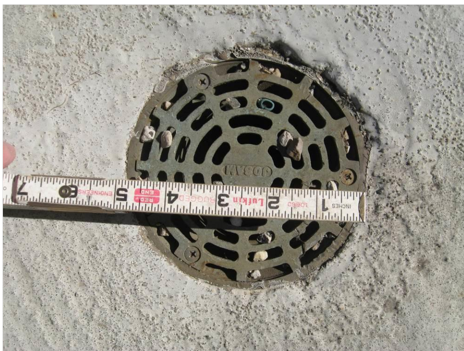
Photo 10 – typical inadequate size floor drain.
