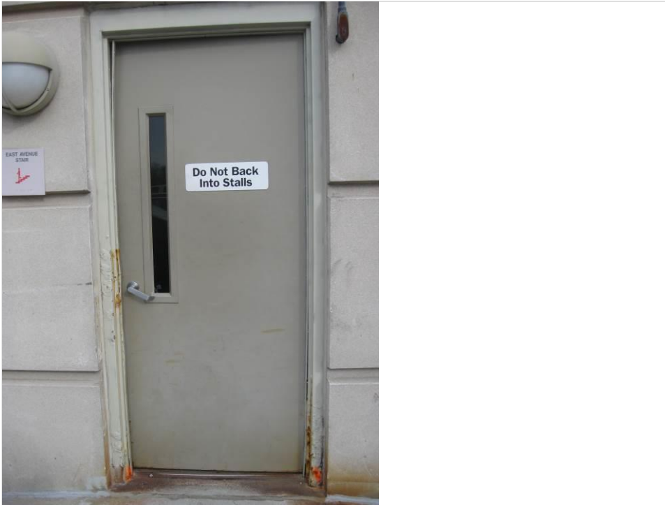
Photo 3 – Severely corroded door and frame.
