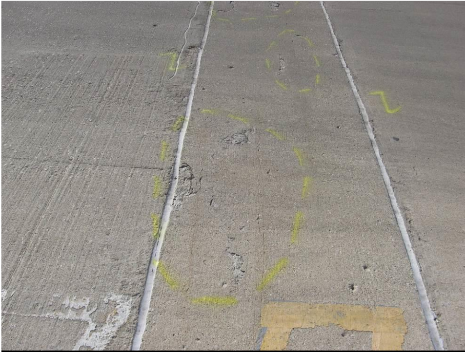
Photo 1 – Typical concrete delamination and cracking in floor slabs at pour strips.
