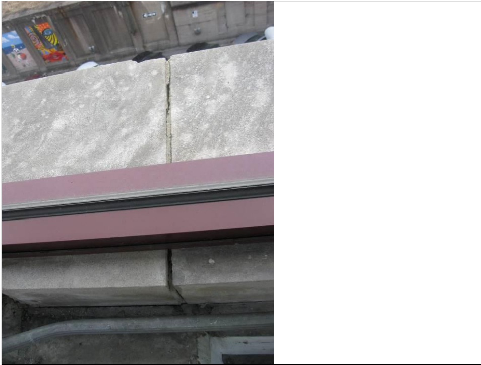
Photo 5 – Severely deteriorated mortar joint under window mullion on stair tower.
