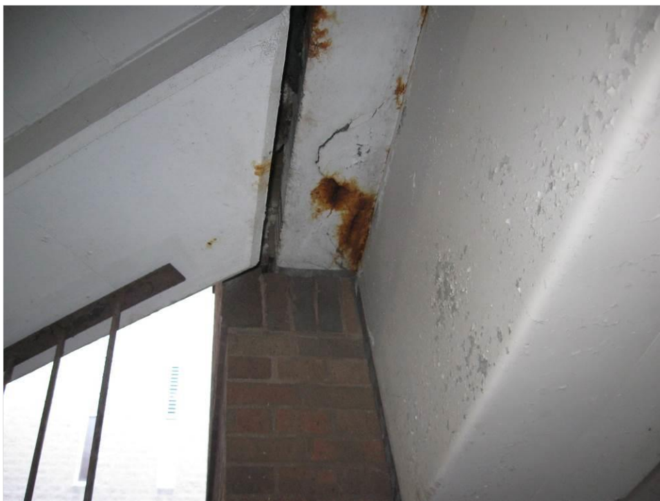
Photo 8 – Typical delaminated beam at stair tower.
