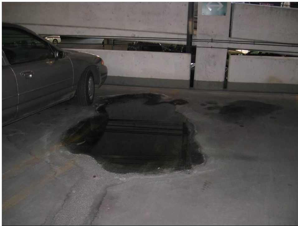
Photo 11 – Area of ponding water of supported slab.
