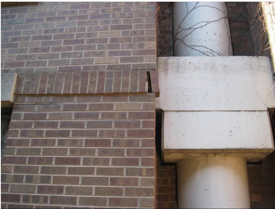
Photo 18 – Loose masonry on façade.
