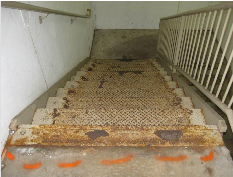
Photo 2 – Corroding stairs within stair tower.
