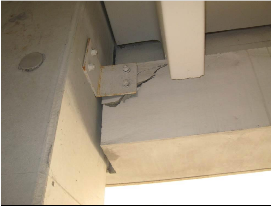
Photo 7 – Broken connection on façade panel.
