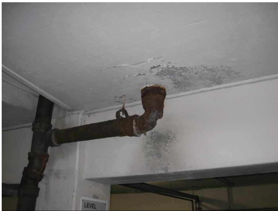
Photo 12 – Broken elbow on floor drain.
