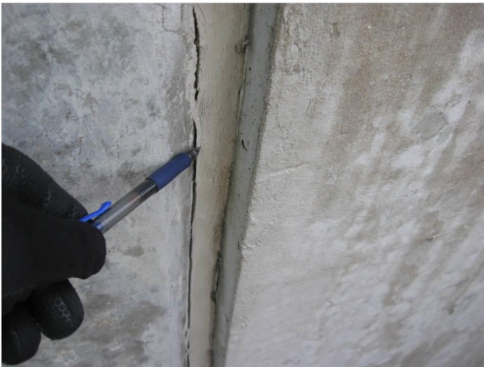
Photo 12 – Typical severely deteriorated vertical joint sealant at perimeter wall.
