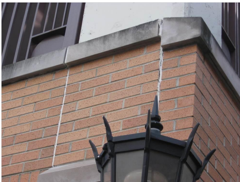
Photo 14 – Severely deteriorated vertical joint sealant on exterior masonry wall.
