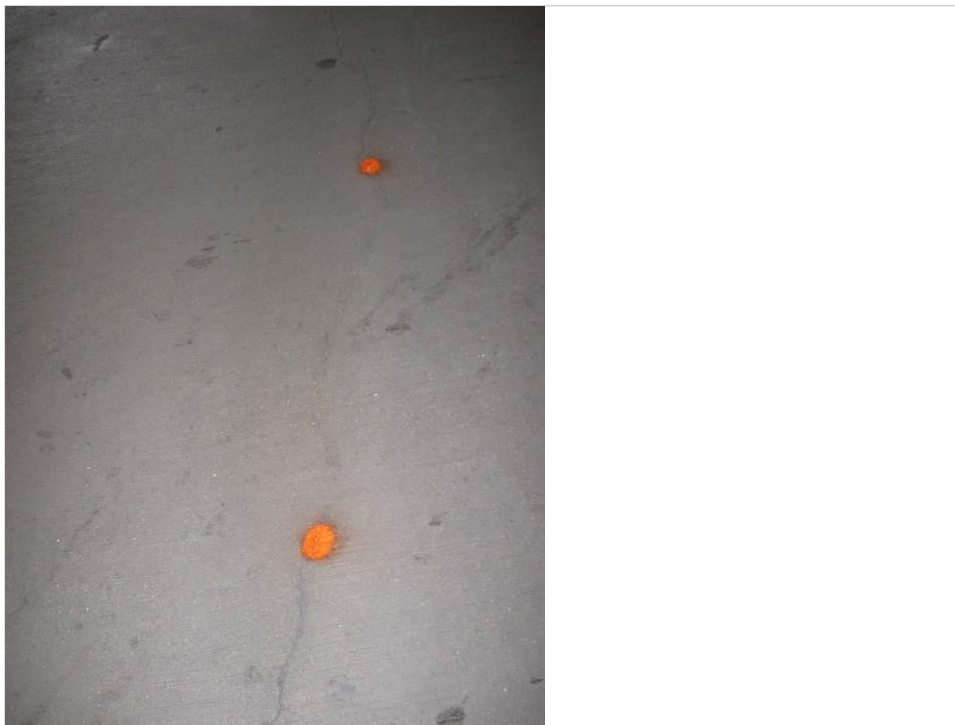
Photo 2 – Typical random floor crack in floor slab.
