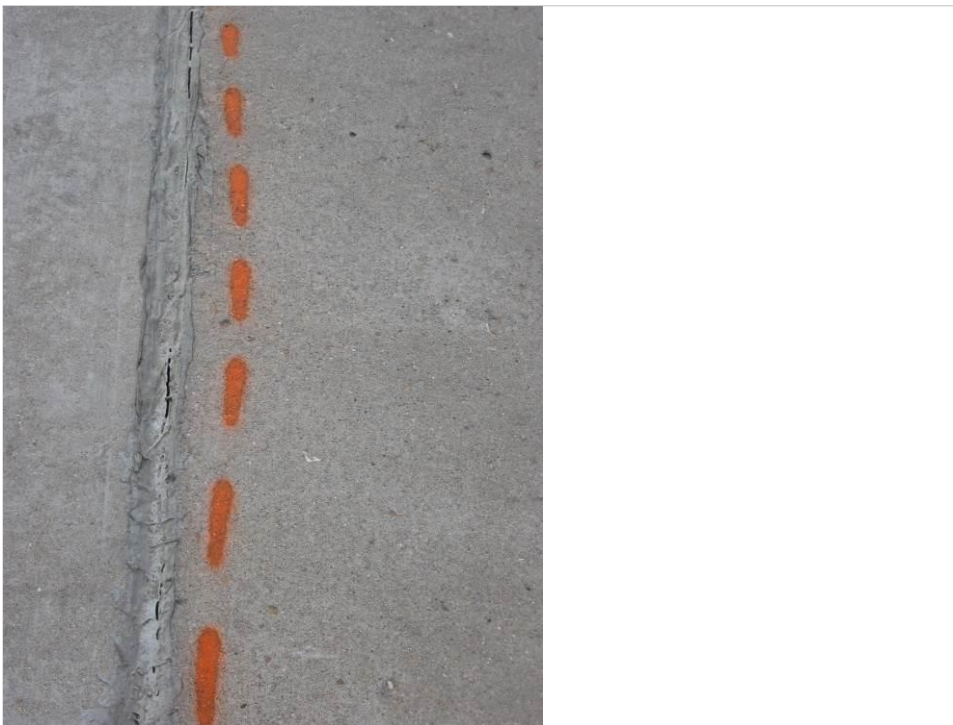
Photo 10 – Typical severely deteriorated tee-to-tee flange joint sealant.
