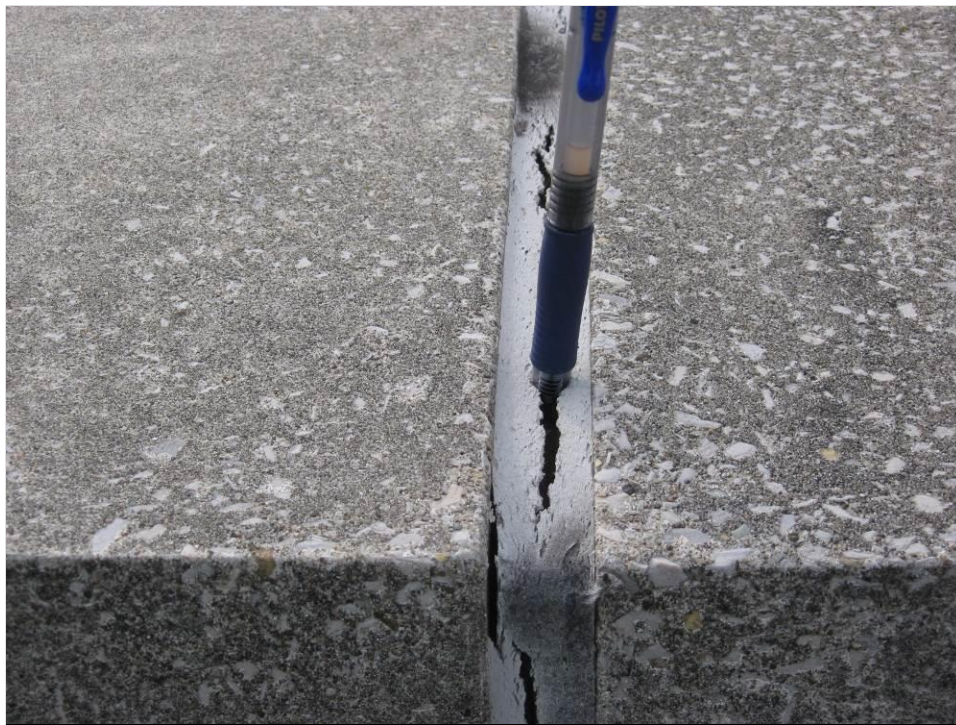
Photo 13 – Typical severely deteriorated cap stone joint sealant.
