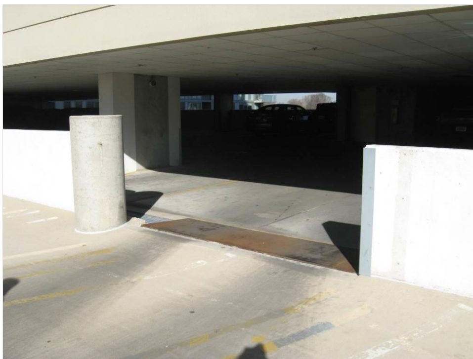
Photo 4 – Open gap area between both structures.
