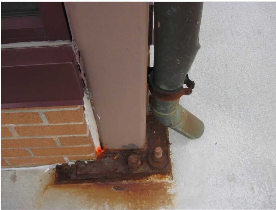
Photo 6 – Severely deteriorated vertical joint sealant on stair/elevator tower.
