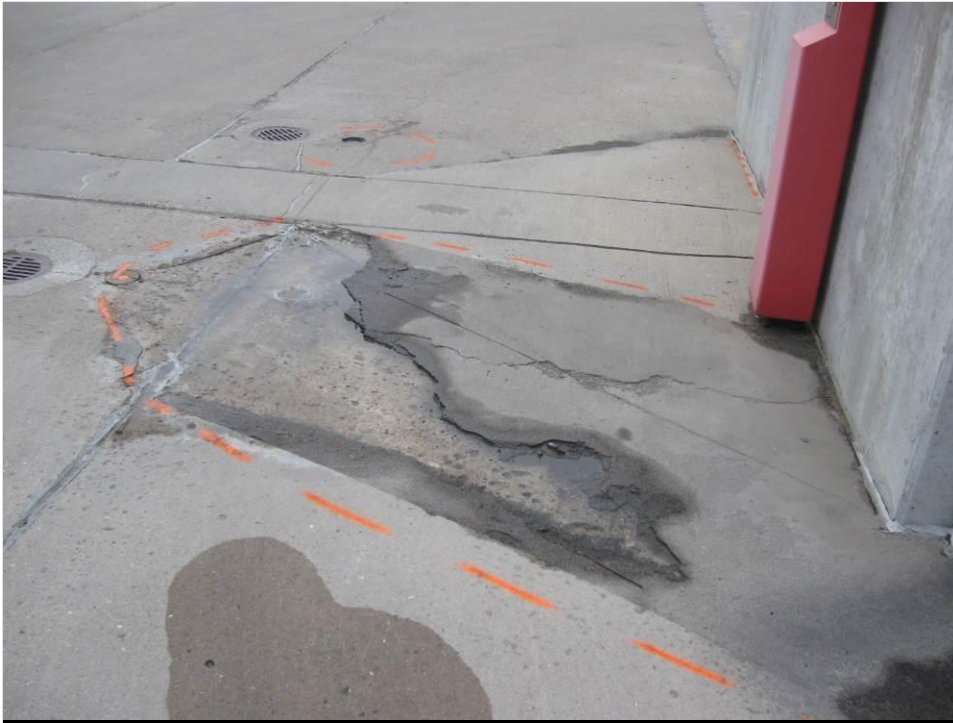
Photo 1 – Typical concrete delamination and spall at cast-in-place wash area.
