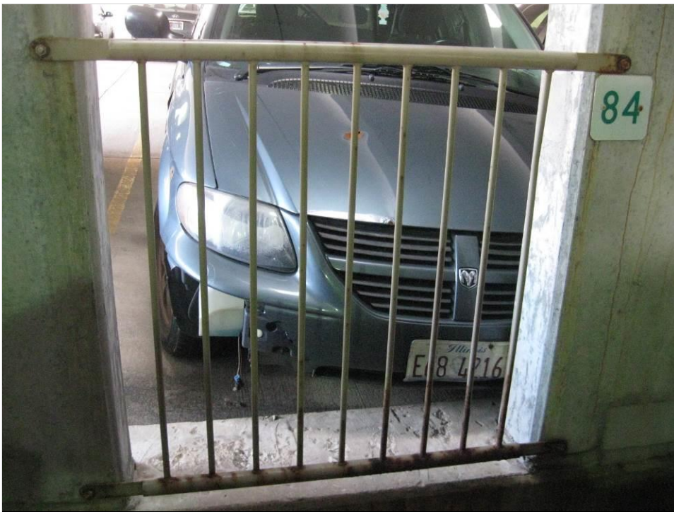
Photo 6 – Typical corroding guard rail on light wall.
