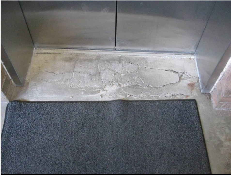
Photo 5 – Floor slab deterioration at elevator landing.
