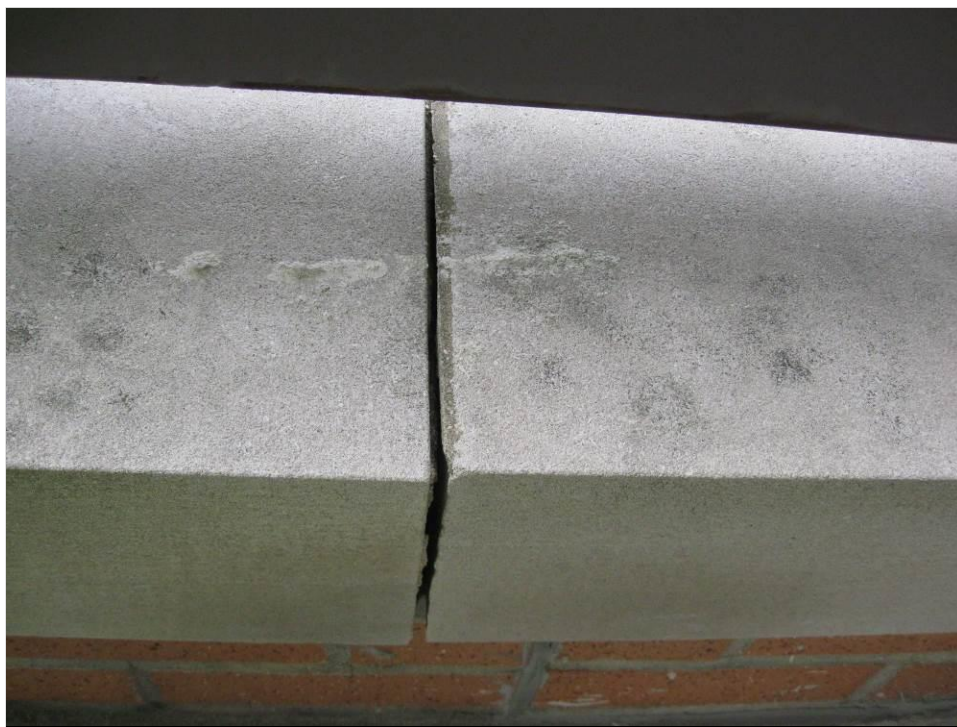
Photo 4 – Typical severely deteriorated mortar joint on cap stone.
