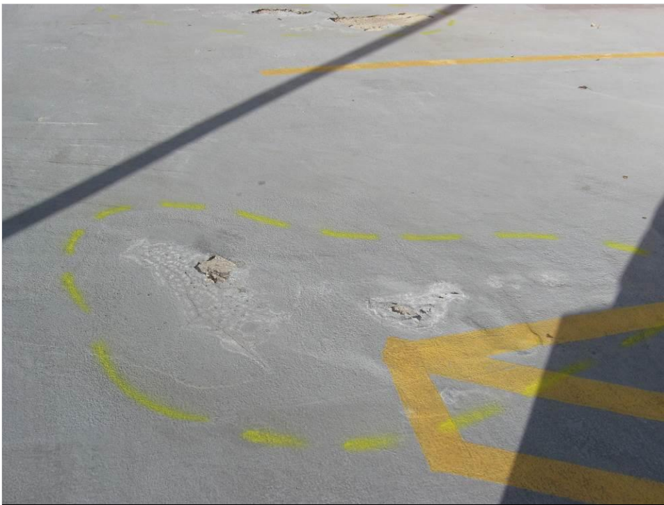
Photo 2 – Concrete deterioration in floor slab under traffic topping.
