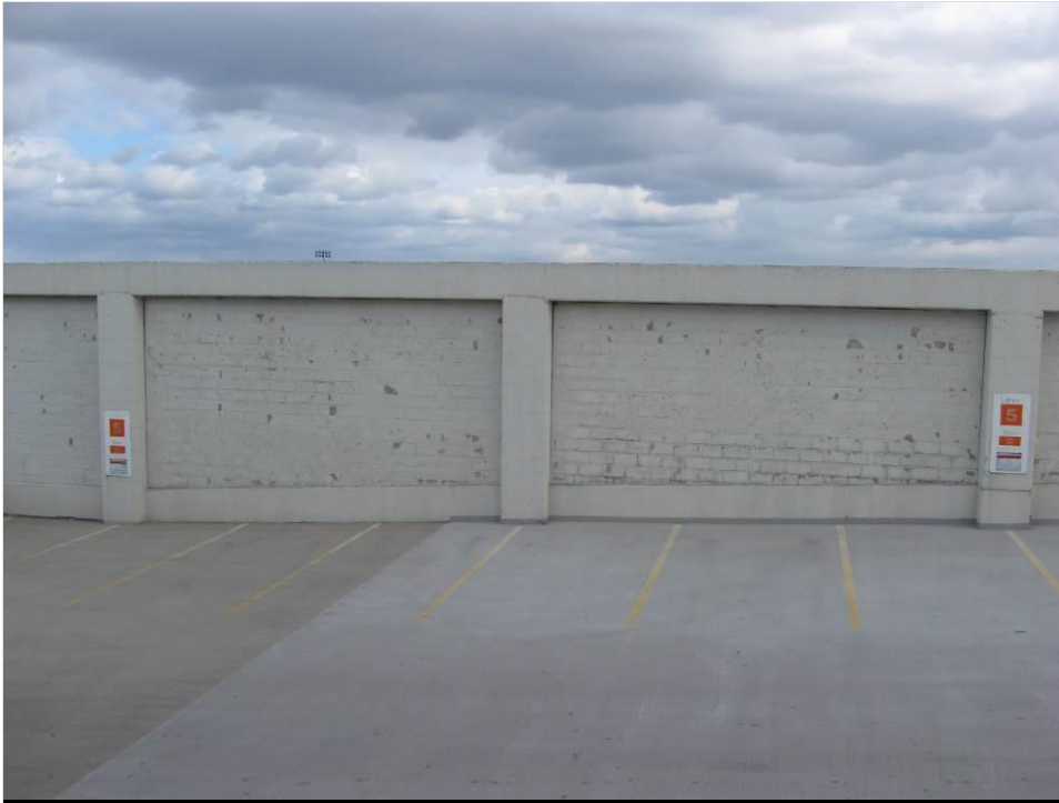
Photo 7 – Severely deteriorated painted masonry wall at Roof Level.
