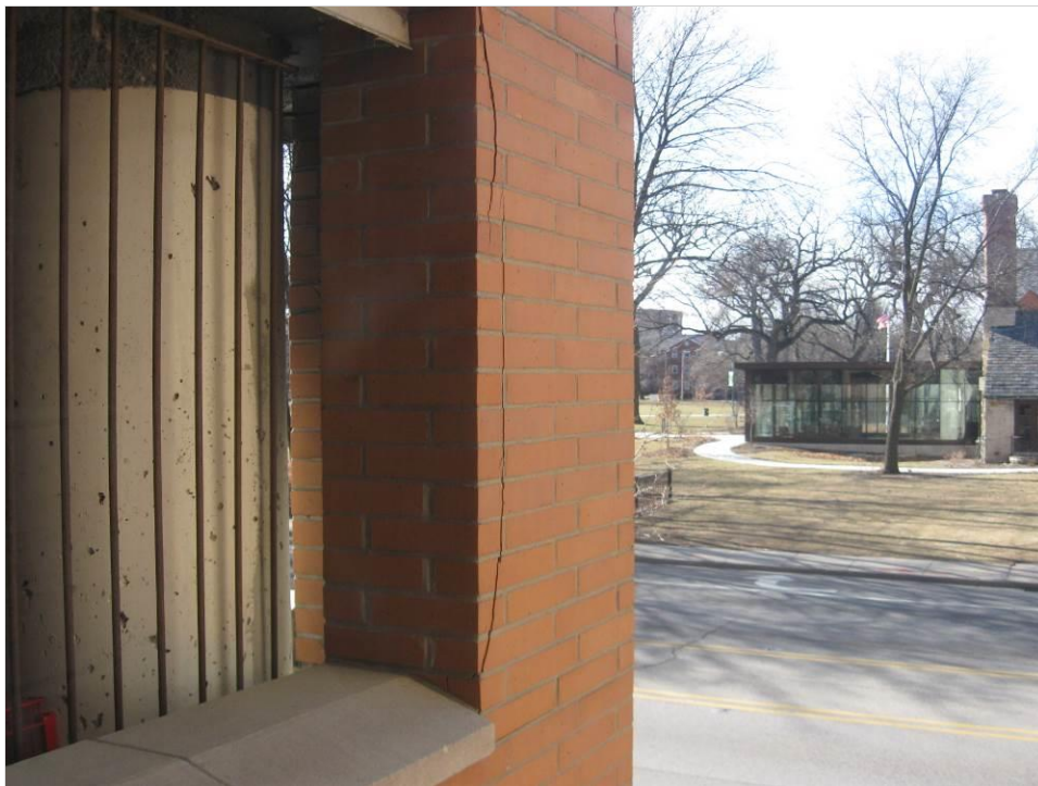
Photo 16 – Crack in masonry façade.
