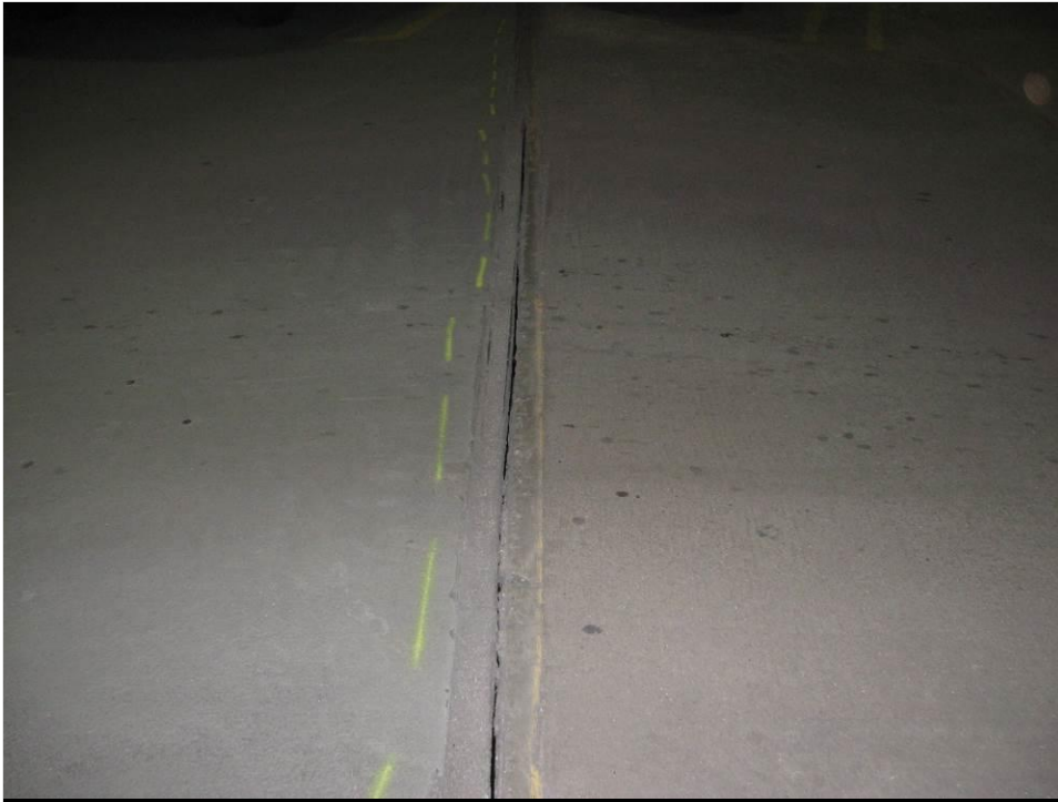
Photo 9 – Severely deteriorated expansion joint on Second Floor.
