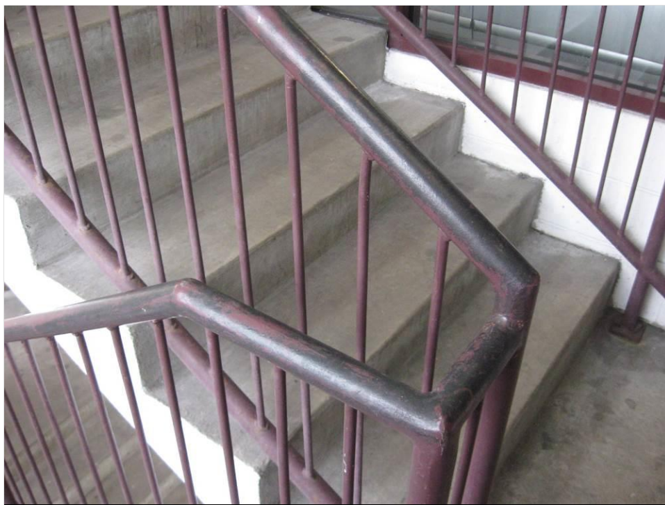
Photo 11 – Worn off paint on stair tower handrails.
