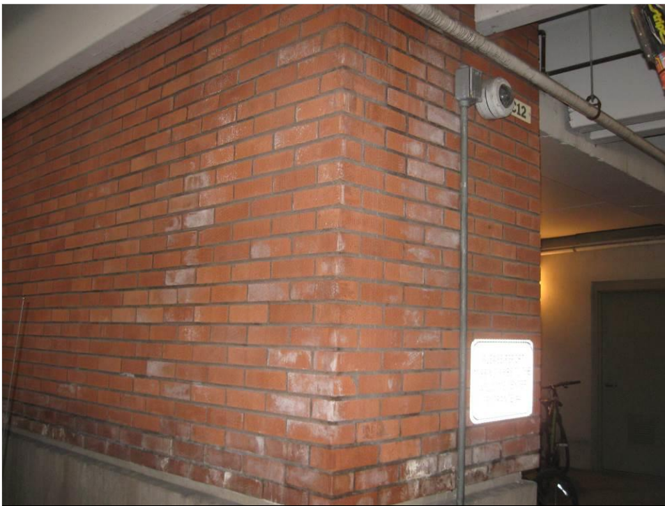
Photo 10 – Efflorescence on masonry due to water infiltration.
