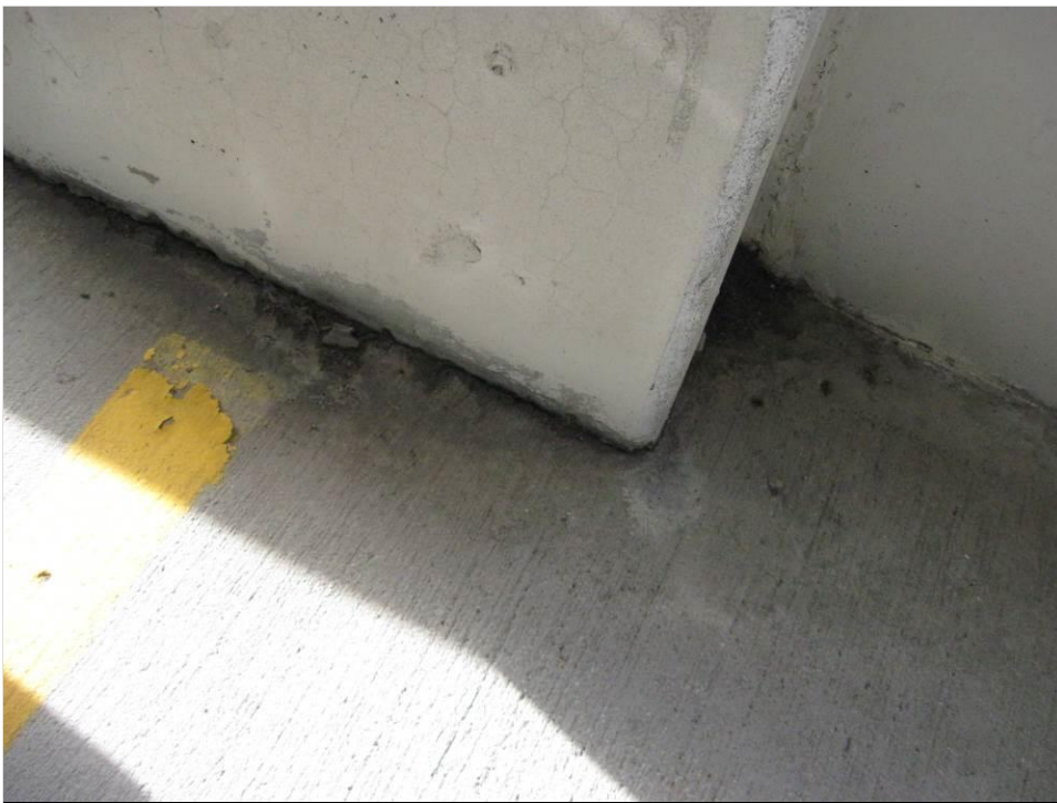
Photo 8 – Typical, no cove sealant between column and floor slab.
