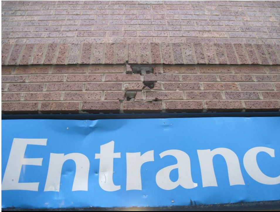
Photo 15 – Damaged masonry façade at entrance.
