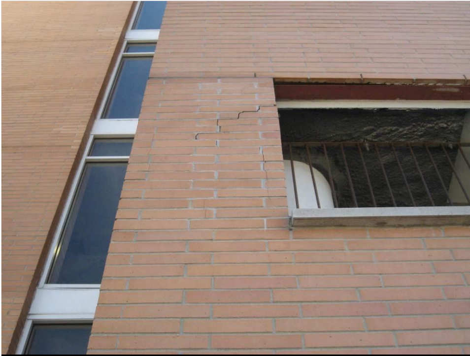
Photo 5 – Crack in masonry on façade.
