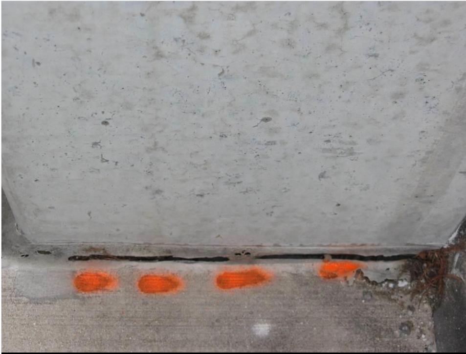
Photo 11 – Typical severely deteriorated cove sealant around column.
