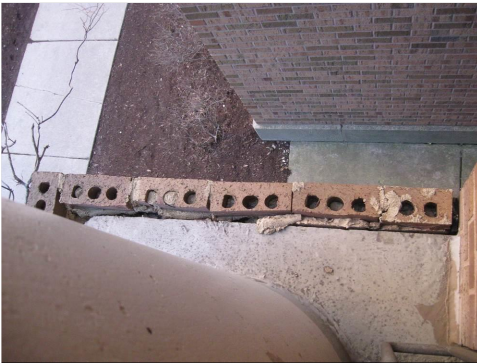
Photo 14 – Masonry wall without any cap stones.
