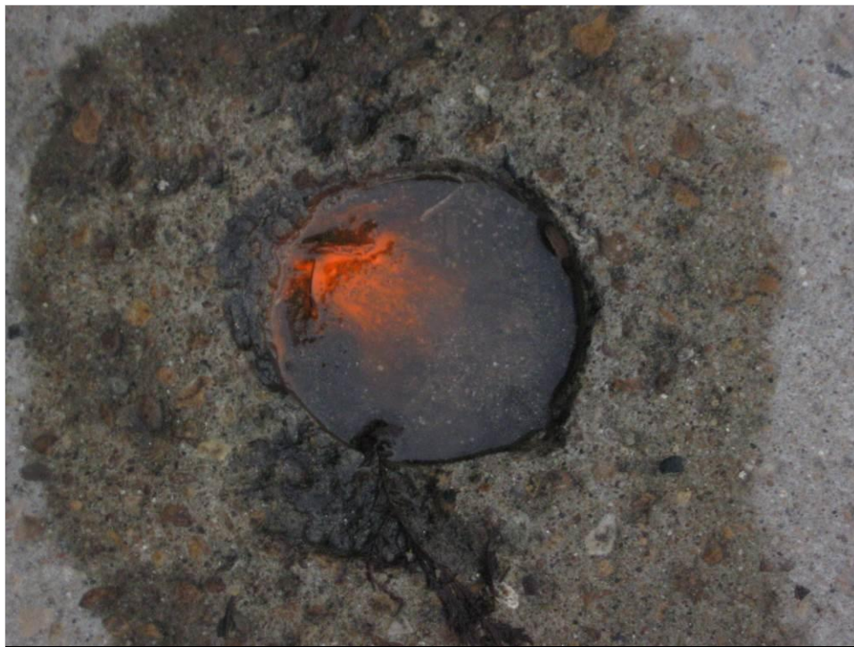
Photo 3 – Floor delamination over lifting loop.
