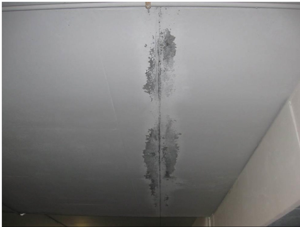
Photo 3 – Active leaking construction joint seen from below slab.
