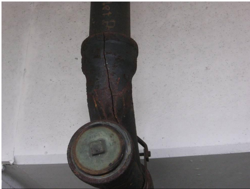
Photo 9 – Crack in drain pipe.
