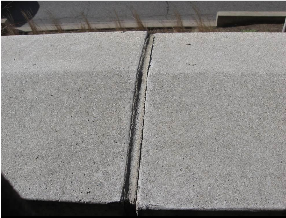
Photo 17 – Severely deteriorated mortar joint on cap stone.
