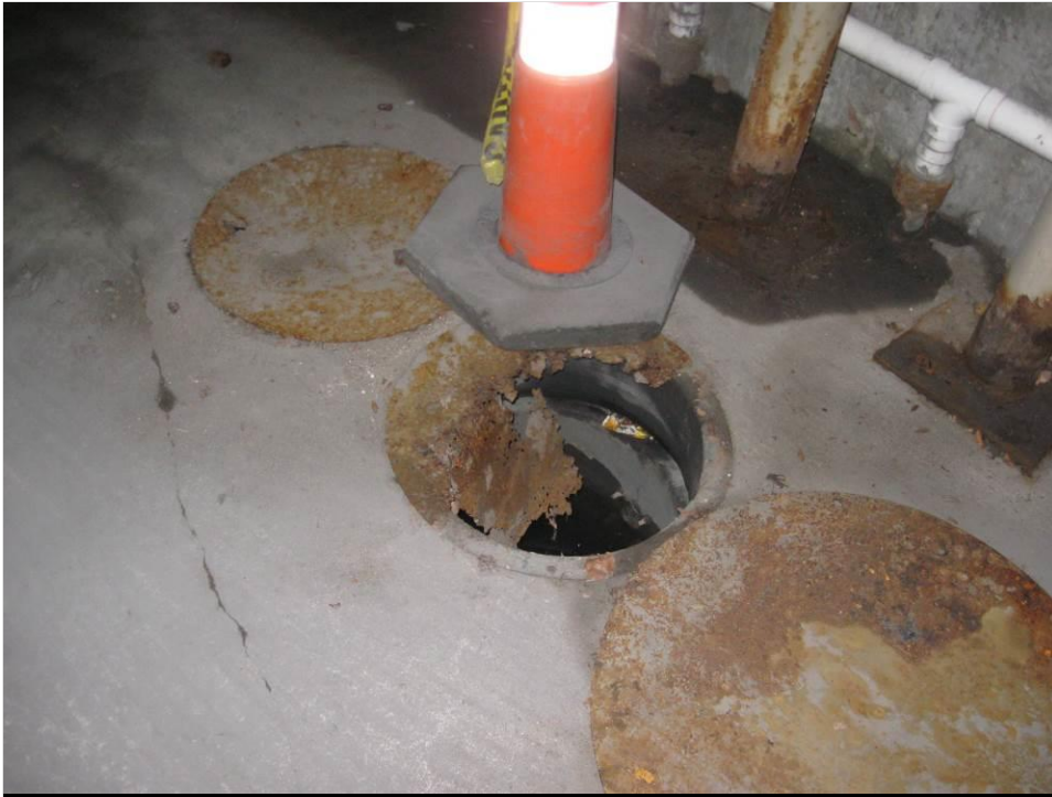
Photo 5 – Corroded cover on triple basin.
