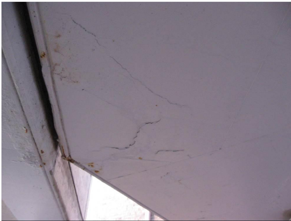
Photo 7 – Typical ceiling delamination.
