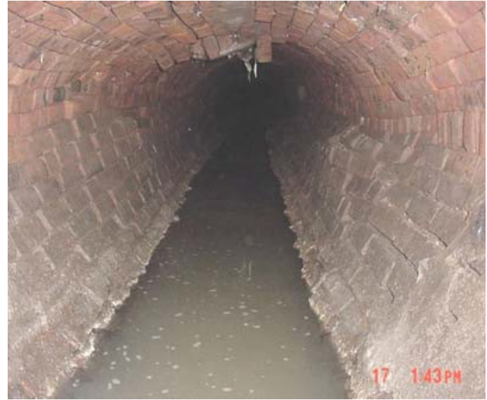
Figure 4. Example of Condition Grade 4 Brick Sewer - Sewer- Collapse Likely in Foreseeable Future
