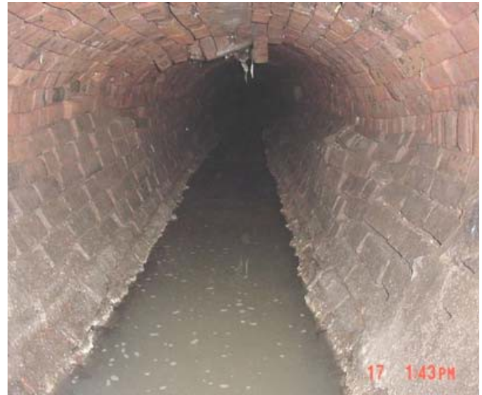
Figure 4. Example of Condition Grade 4 Brick Sewer - Sewer- Collapse Likely in Foreseeable Future
