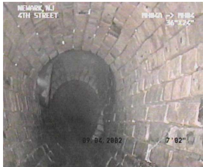
Figure 2. Example of Condition Grade 2 Brick Sewer- Minimal Potential for Short-Term Collapse; Further Deterioration Probable
