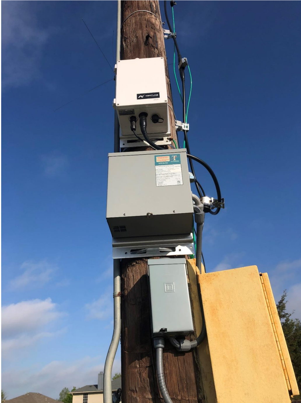
UPS and Gateway mounted on wooden pole.
