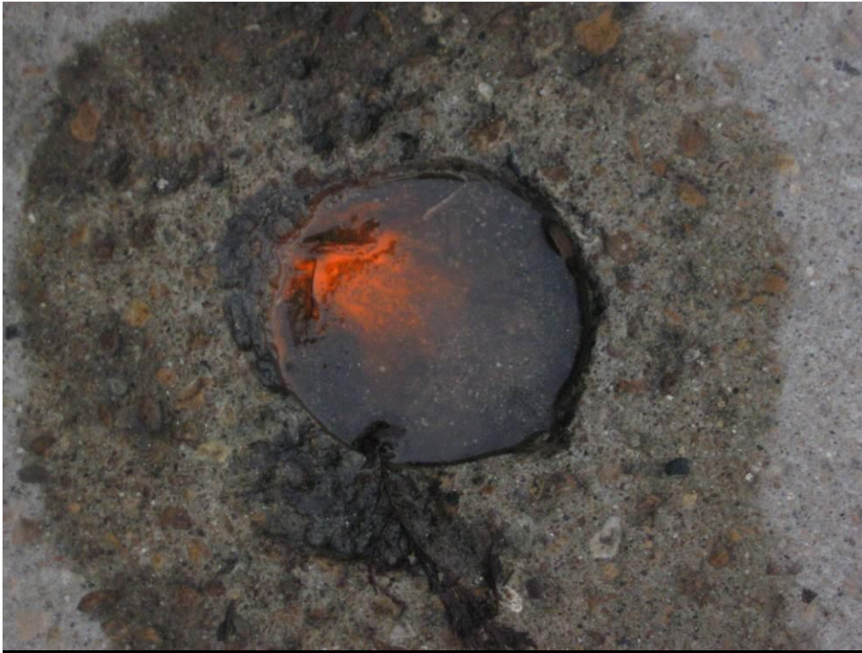
Photo 3 – Floor delamination over lifting loop.
