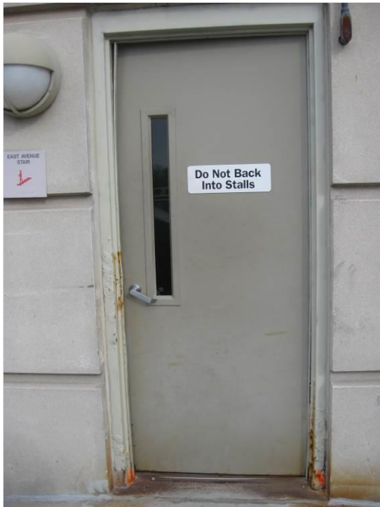
Photo 3 – Severely corroded door and frame.
