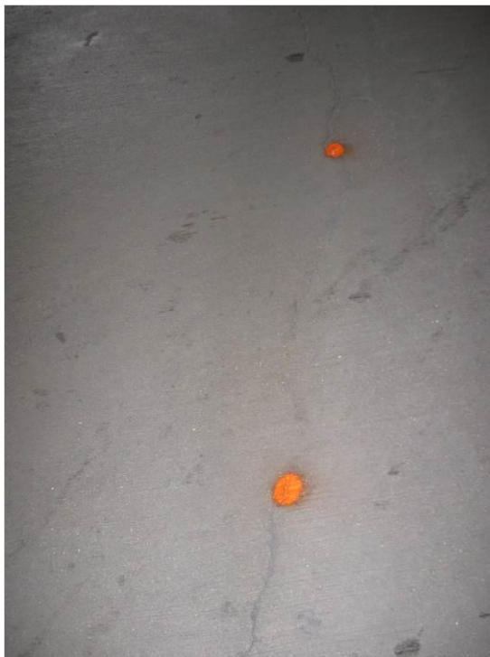
Photo 2 – Typical random floor crack in floor slab.
