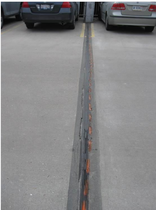
Photo 14 – Severely deteriorated expansion joint at grade slab.
