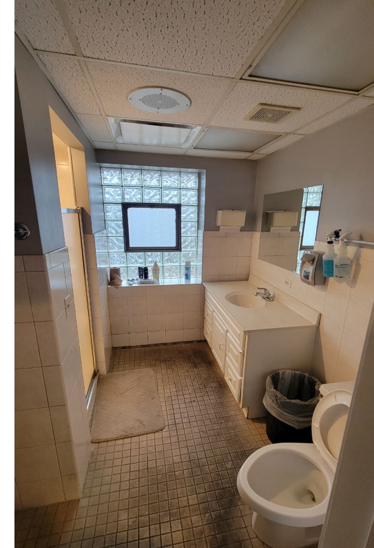
INSUFFICIENT TOILET FACILITIES
